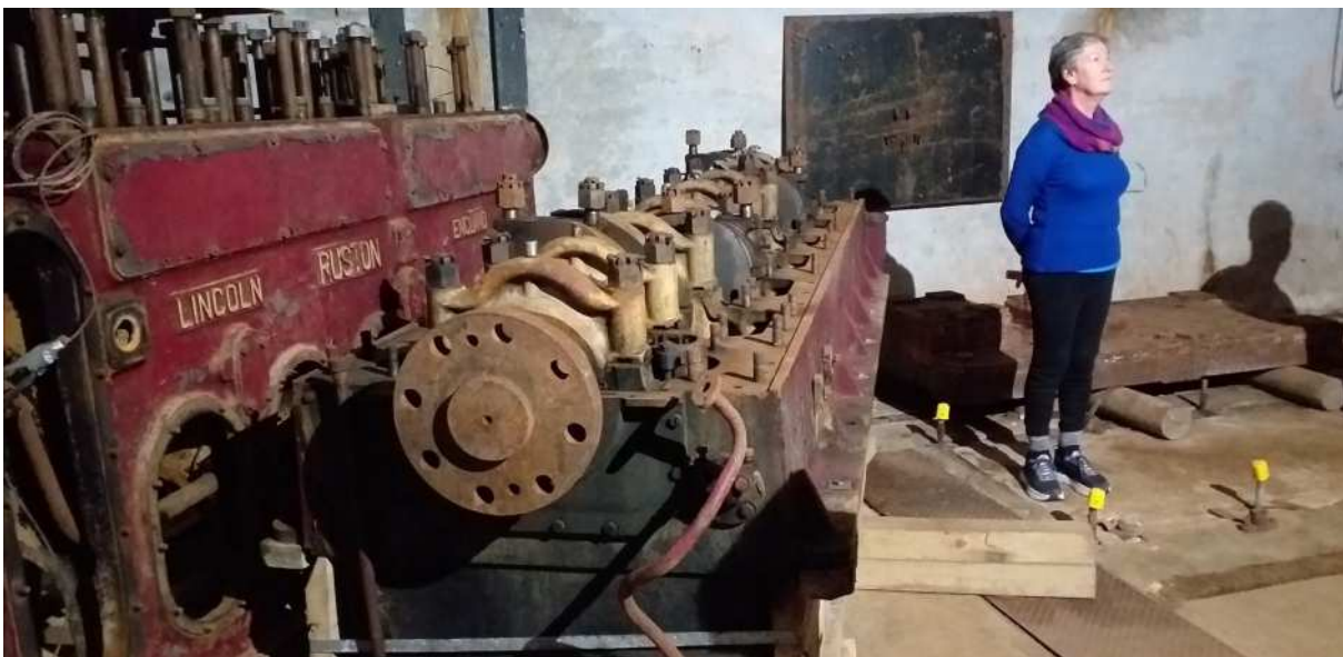
Ruston Hornsby crankcase lying beside its cylinder block deep underground at Stony Batter.
